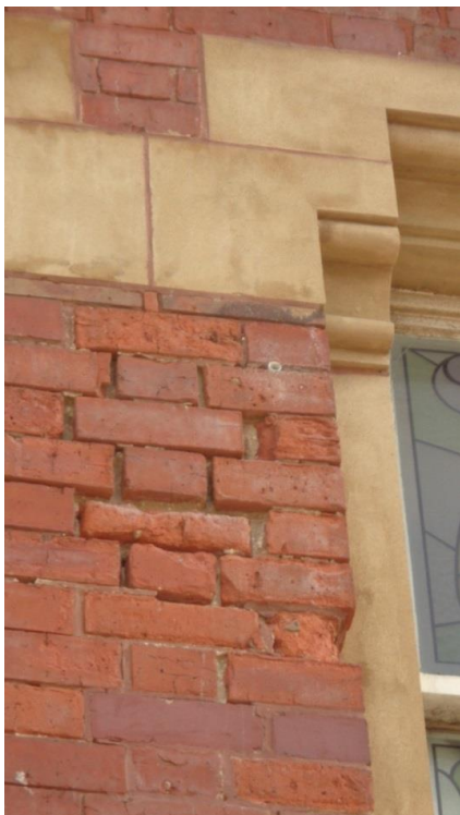
Late Victorian building repointed with cement mortar which has led to frost damage
